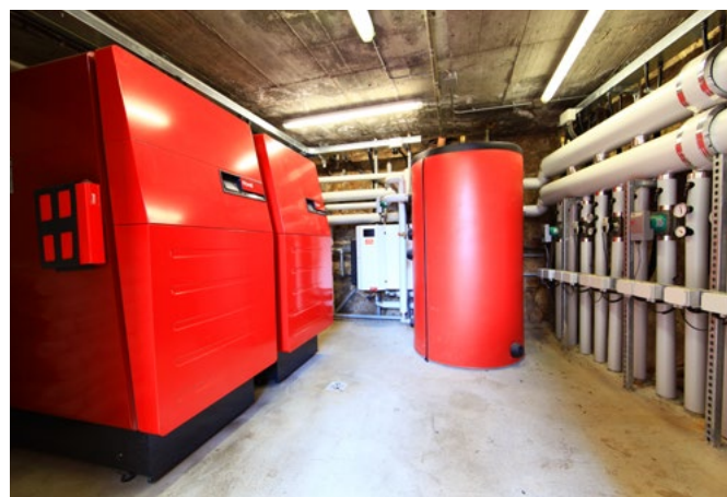
A complete solution from Hoval supplies the Cappuccini Resort with heating and domestic hot water.
