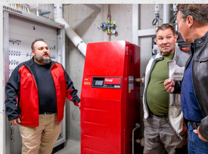
The 1500 m 2 living space is heated using an UltraGas® 50 gas condensing boiler combined with an ESSR 100 calorifier.
