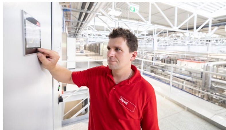
The energy-optimised dehumidification control system guarantees the required air quality in the Spitz production hall.
