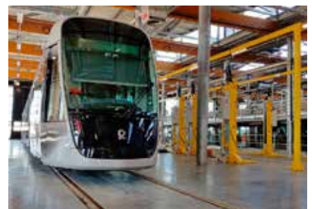
Using TopVent® decentralised air circulation units in a tram maintenance hangar.
