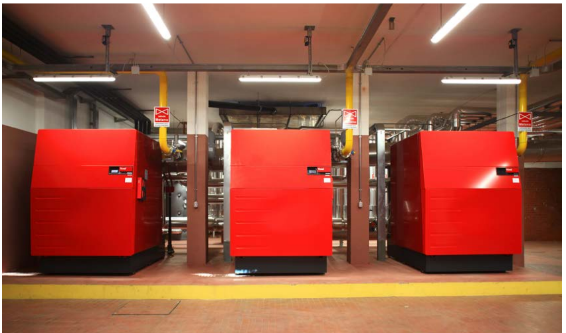
Three UltraGas® condensing boilers supply the site network with heat for heating and hot water.
