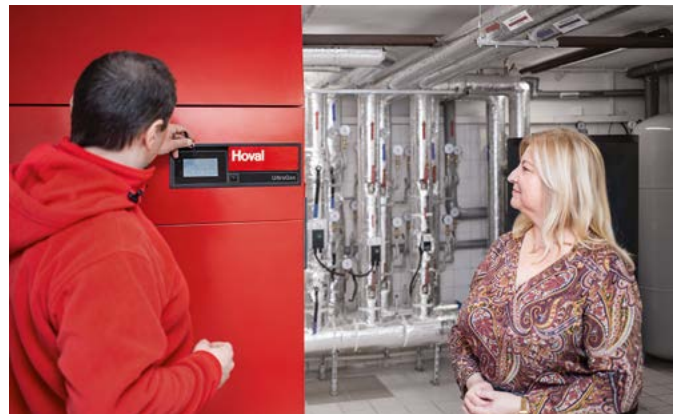
Project Manager Michał Duliban and Head of School Elizabeth Klaczak-Łach in the school’s boiler room.
