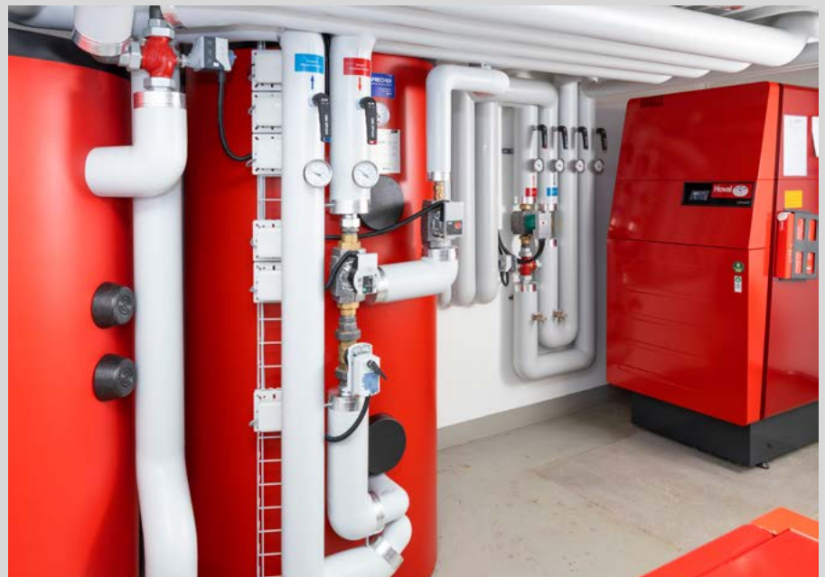
Two UltraSource® air/water heat pumps, an UltraOil oil-fired condensing boiler, the CombiVal CR 800 domestic water storage tank and an EnerVal 800 buffer storage tank created the perfect hybrid solution.
